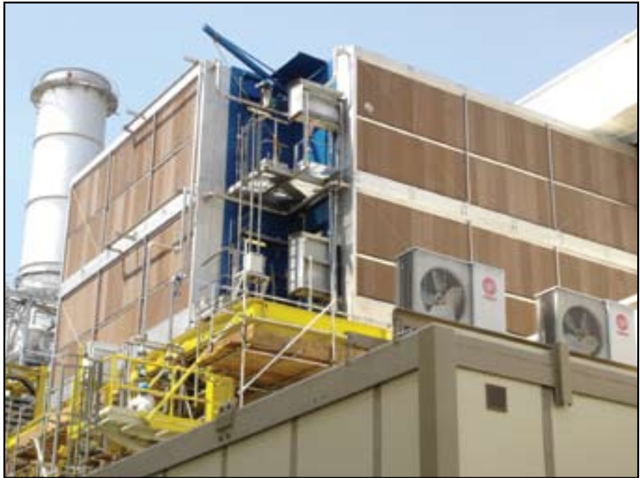
Evaporative air cooler. Photo of installation being made during scheduled 5-day gas turbine inspection outage. Three-sided design meets structural codes for power stations to withstand 200 kph winds and earthquakes up to magnitude 8.
