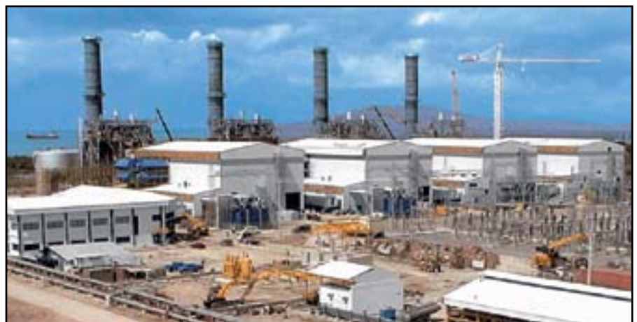
Santa Rita 1000-MW station. The first of two combined cycle stations at Batangas, on the main Philippine island of Luzon, built around four V84.3A single-shaft combined cycle power blocks rated 250 MW and 56.8% efficiency each at 32°C sea level and 80% relative humidity site conditions, on natural gas fuel. The gas turbines have been retrofitted with evaporative air inlet cooling to enhance hot day performance.
