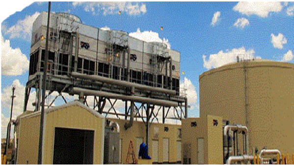
Chillers Building and TES TANK
